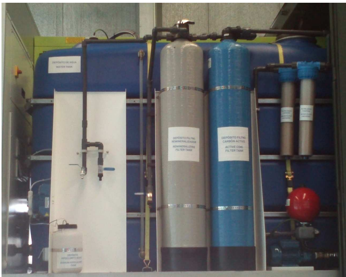
Water treatment system
